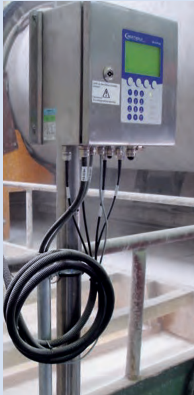
MicroPolar installation in a power station for measuring the concentration of a limestone suspension
